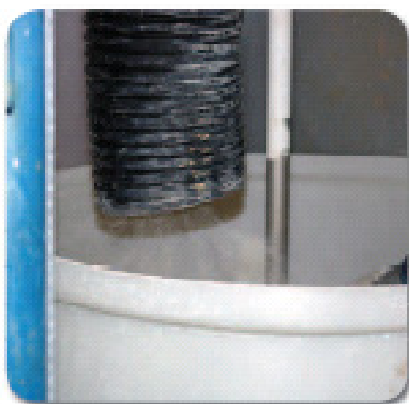
Local exhaust ventilation controlling fugitive emissions during precursor mixing at a primary nanoscale metal oxide production facility.
